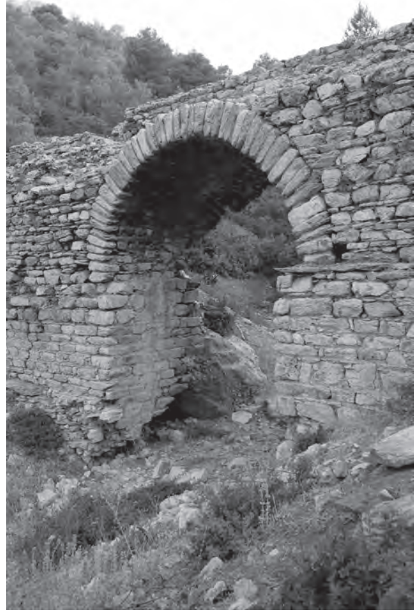
Fig. 3. Adamtoluboğaz aqueduct-bridge with an illicit excavation in the background.
