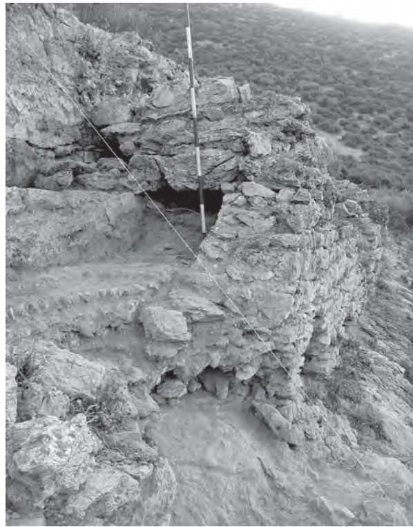
Fig. 5. Supporting pillar 17 in section XI. Type II stands on a covering slab of the older Değirmendere line, of which the substructure of the base of duct is clearly visible. Above: wall type C of the younger line.
