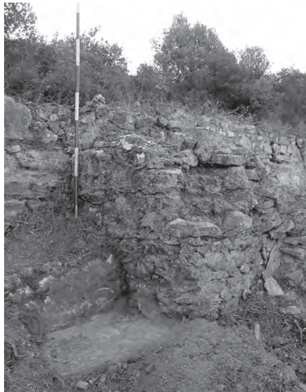
Fig. 8. Supporting pillar 26 in section XI, type I which is built into the channel of the older line.
