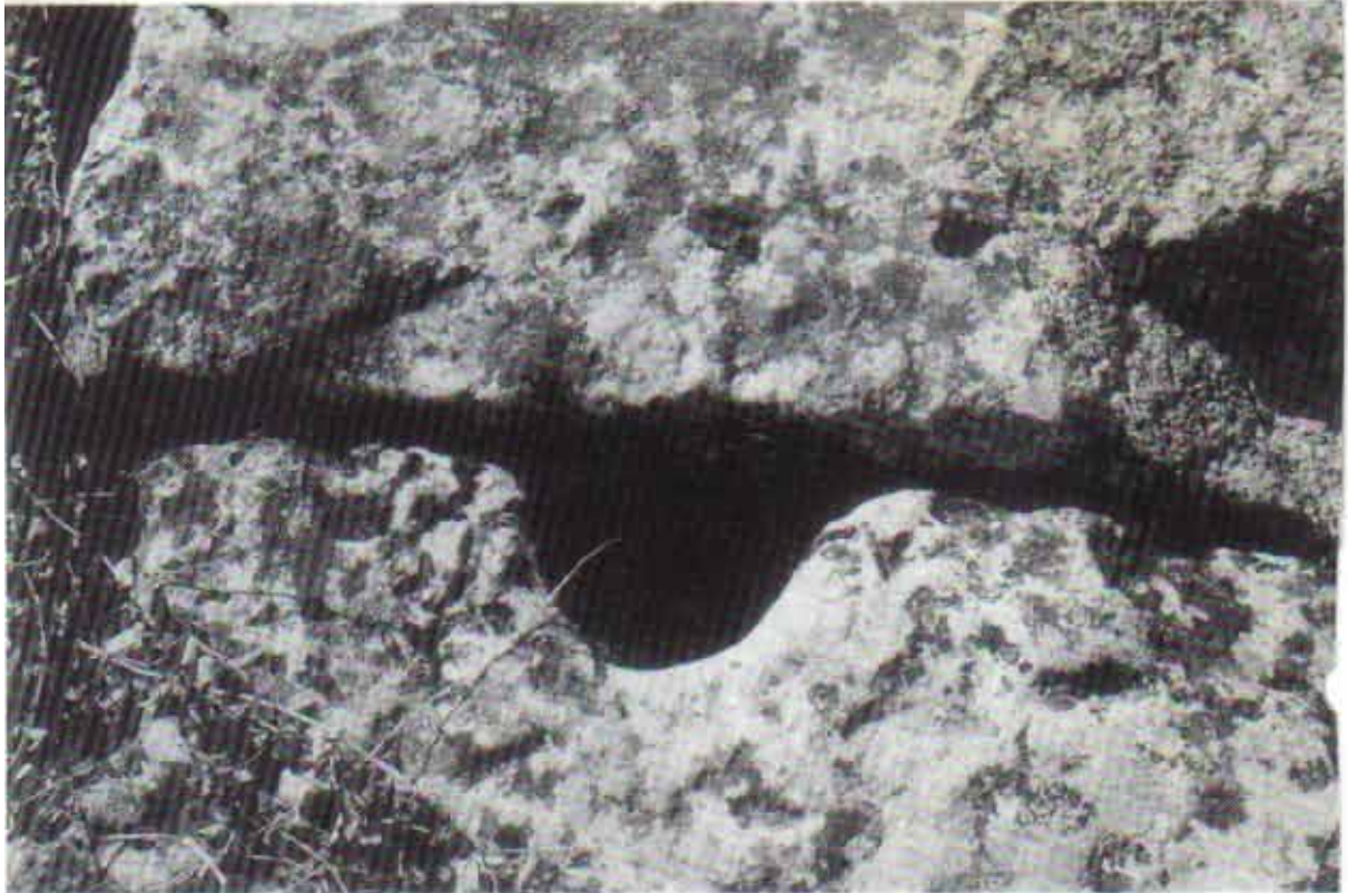
2 a. Laodikeia: hole drilled in joint between blocks of stone pipeline (Fahlbusch)
