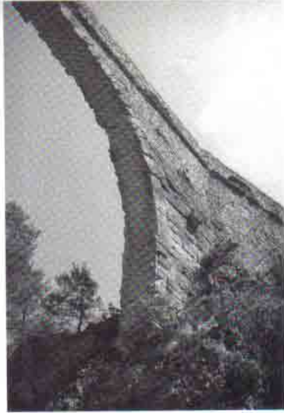
Fig. 16 Detail of the southeast abutment, southwest face, and bend in the bridge. View to southeast. Dia Troia 42480.
