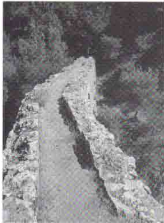
Fig 18 The open water channel on the deck of the bridge. View to south. Dia Troia 42463.
