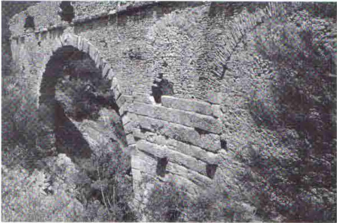
Fig. 17 The southwest face of the bridge. View to the north. Dia Troia 45982.
